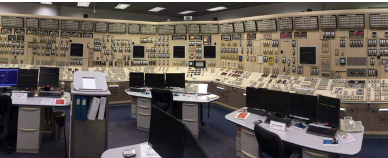
The (simulation) control room at the Shearan Harris Nuclear Power Plant, 2017 (Image by RadarMan under CC)
